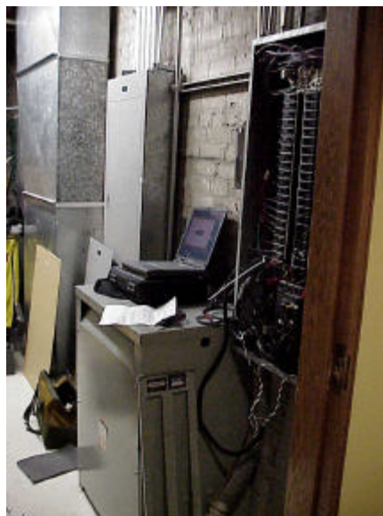
Picture 1 - Electrical Closet, Transformer, and Panelboards
